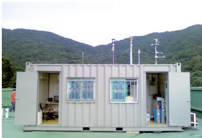
Measuring station for air quality monitoring: among the analyzers installed in this portable building is a MARGA system, which can be operated fully automatically over an extended period of time.
